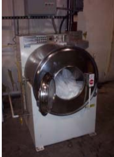
Figure 3. 50 pound Milnor washer/extractor installed at Anovotek, LLC laboratory.
